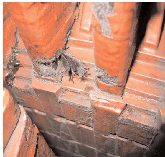
Impact damage: It may be possible to successfully repair damage of this nature.
