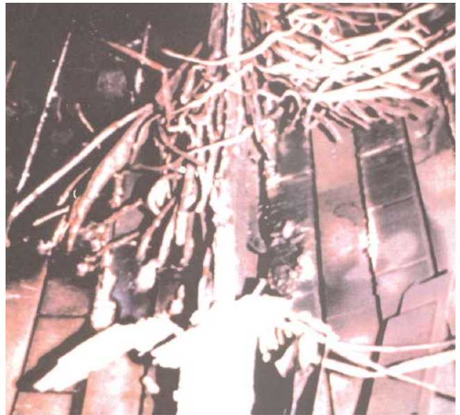
Major electrical fault: "Repair" of this type of damage may not be reasonable or practical
