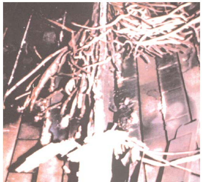
Major electrical fault: "Repair" of this type of damage may not be reasonable or practical
