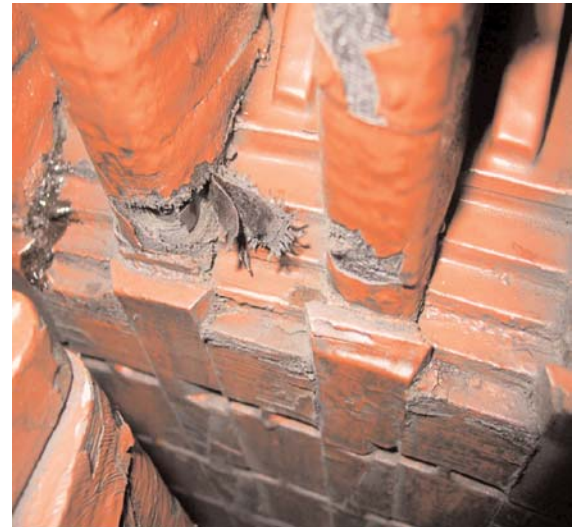
Impact damage: It may be possible to successfully repair damage of this nature.
