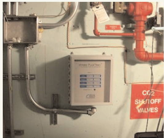
Hydro Flux Monitor mounted on generator wall takes signal from the flux probe and connects to plant LAN. Installation at NYPA's St. Lawrence Power Project.
