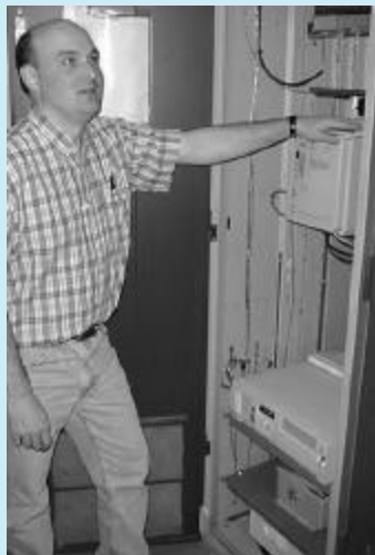
FluxTrac installation at Florida Power & Light, Riviera Plant by Iris's Supervisor of Product Development Mark Susnik
