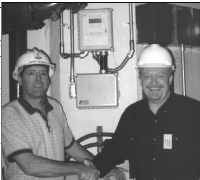
Randy Brawley (Chelan PUD) with Randy Wallman (Iris) in front of a completed HydroTrac installation at Rock Island Dam
