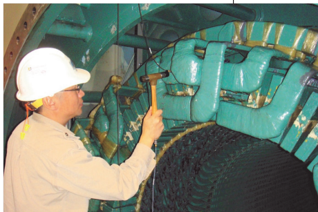
Iris personnel performing a bump test on 200MVA turbine generator
