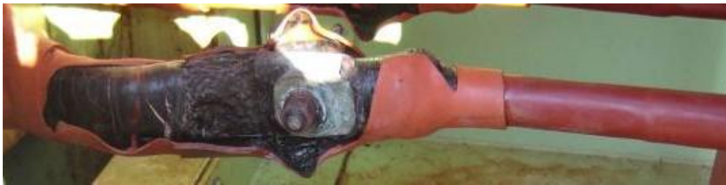
Figure 2. Overheated Connections in Motor Terminals
