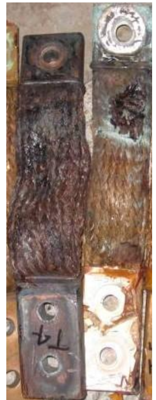
Figure 3. Damaged Flexible Connectors
