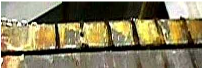
Figure 2. Damage in Bar due to Slot PD Activity
