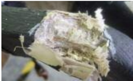
Impact damage to the groundwall insulation exposing the copper strands
